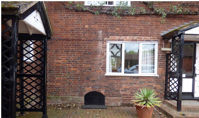
Fig. 3. The SE end of the N range, showing the site of an earlier door, behind the flowerpot, and the coal-shoot for the cellar.
