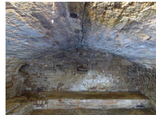
Fig. 5. The cellar N wall, note the blocked openings in the centre of the wall and to the left.
