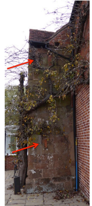
Fig. 11. Side with blocked windows shown by arrows.
