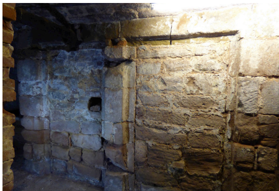
Fig. 7. The two blocked doorways in the W wall of the cellar, note the pintle for the door-hinge on the right frame.
