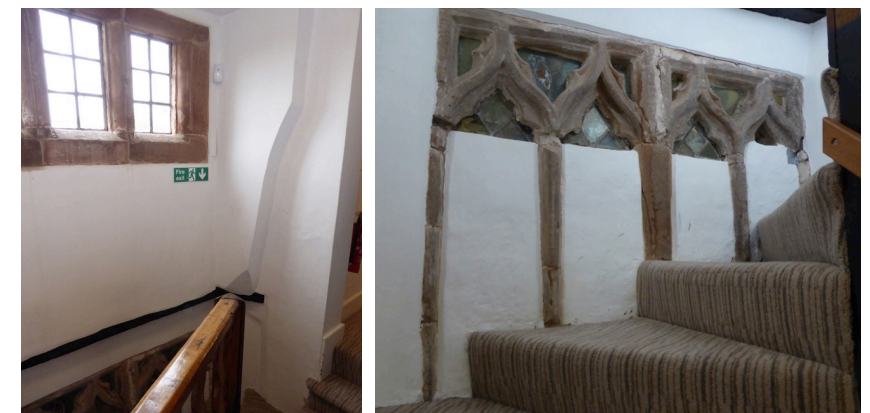
Fig. 12. The staircase, showing the cut-back wall and upper window, left, and pair of blocked windows with glass still in place, right.
