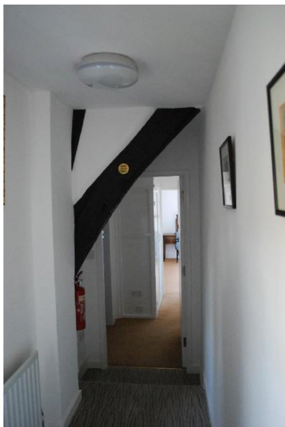
Fig. 6. Arch-brace and post head of remaining timber-framing on the west side of the north range [Photo: James Edgar]
