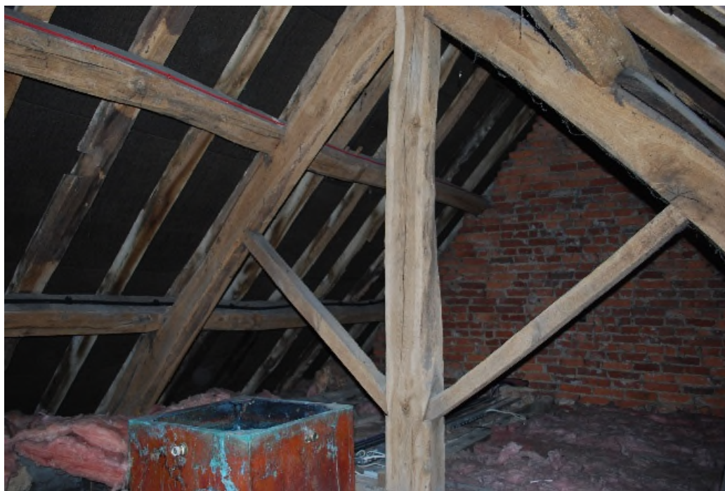
Fig. 4. The roof over North Range, showing some reused smoke-blackened rafters and the 18 th -century king-post roof truss. [Photo: Alex Russell]
