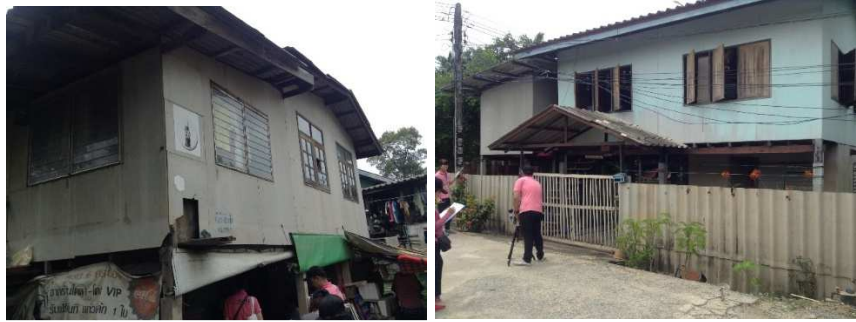
Figure 5.8 Housing features of old houses of central region which homeowners do not have their own land (suburban group).
