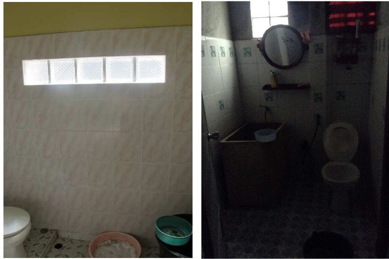
Figure 4.13 Lighting condition of toilets in houses of southern region
