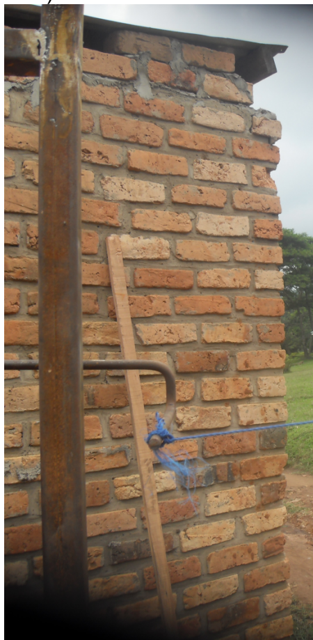
Figure 3 Brick shelter with bad mortar technique
