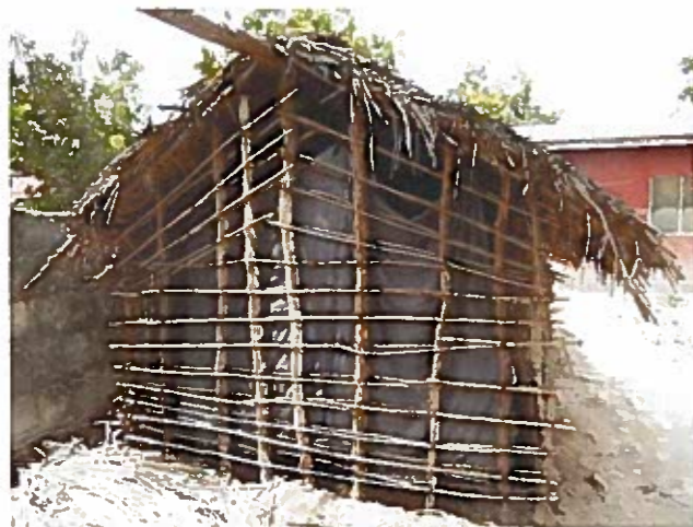
Figure.4. Detail of timber support to a mud House, House 7 (Author)
