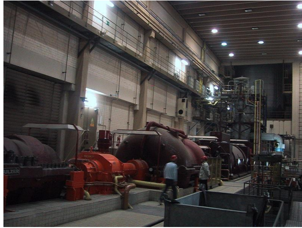
Fig. 6 A view of the power house at the Huntorf CAES plant [17]
