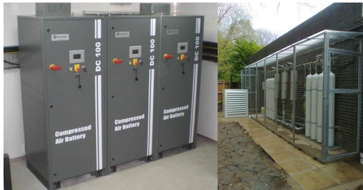
Fig. 10 A CAB back-up power system for a Cooperative Bank building in Stockport U.K.
