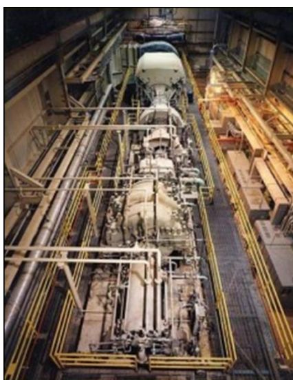
Fig. 8 The compressor, generator/motor and turbine train in the McIntosh CAES plant [16]
