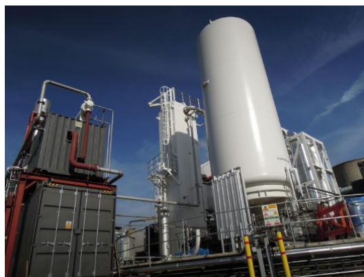
(a) A view of the Highview pilot liquid air energy storage facility
