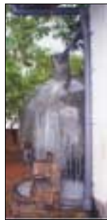
Simple downpipe first flush system in Sri Lanka (Picture: T. Ariyananda)
