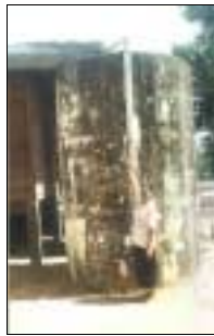
Poorly designed first flush system which cannot be operated by the user
