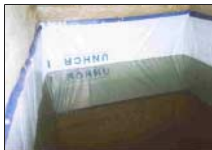
Tarpaulin lined underground tank in rural Uganda (Photo D. Rees)
