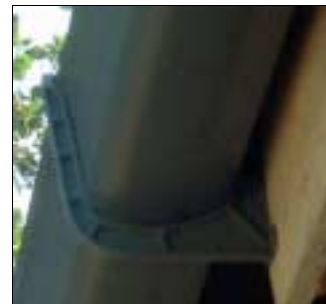
Plastic brackets mounting gutter to fascia board in Sri Lanka (Picture: B. Martinson)
