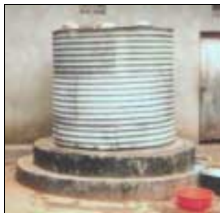
A corrugated steel tank in rural Uganda - note the concrete ring around the bottom repairing leaks (Picture: D. Rees)
