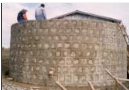
A communal masonry tank in Rural Ethiopia (Picture Water Action)
