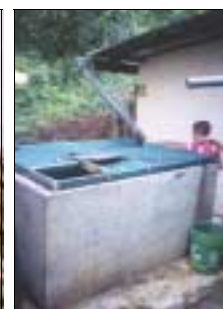
A plastered rectangular brick tank in rural Sri Lanka (Picture: D. Rees)
