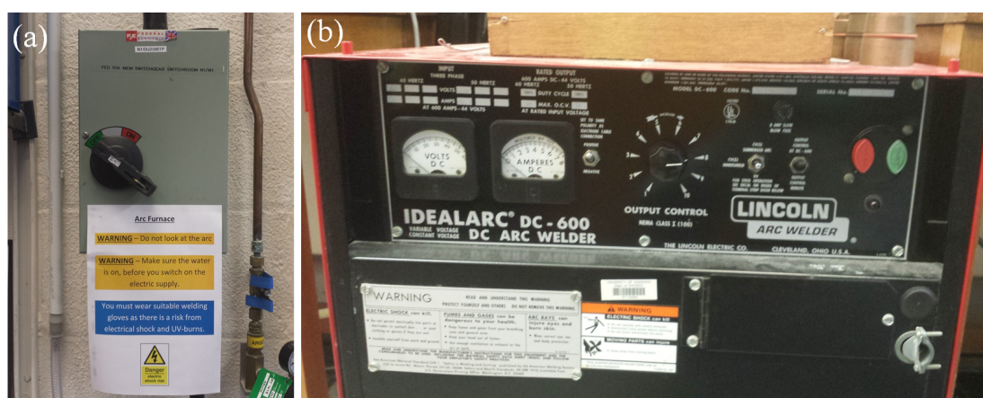
Figure 7: (a) Power source for the welding unit and (b) control panel for the welding unit.
