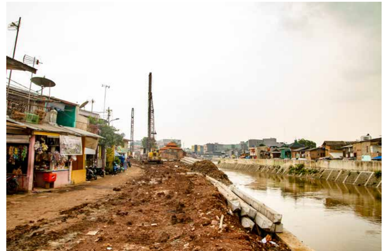
The space left by demolished homes along the Ciliwung riverbank in the Bukit Duri neighbourhood.
