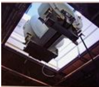
Picture 7. The open MRI is lifted out of the roof of the Interventional Centre.
