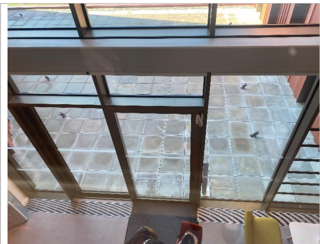
Main access door from lobby on the third floor shows key and Salto access.
