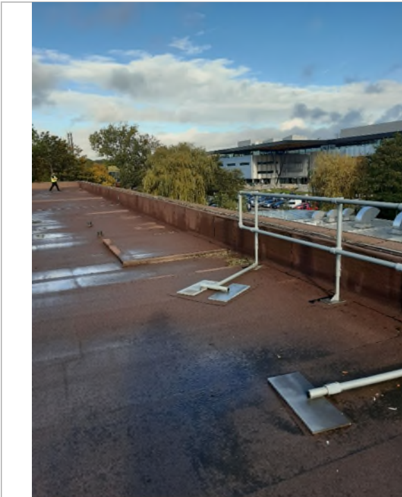
Missing guard rail
