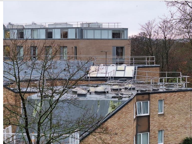
Sky lights and edge protection and roof incline with latchline system
