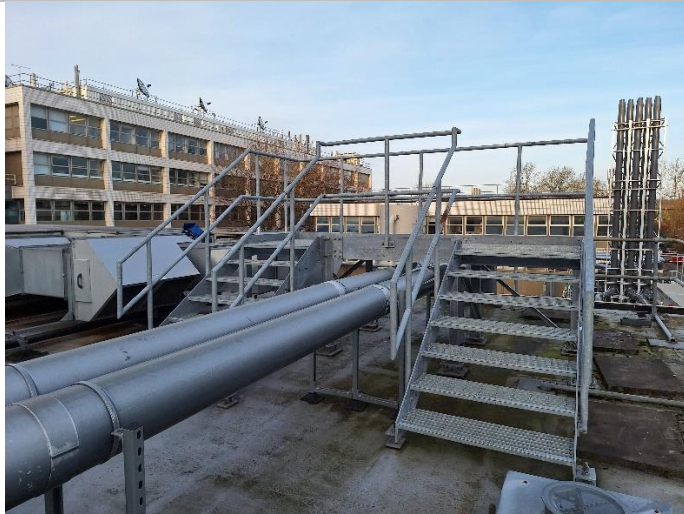
Gantry over pipework
