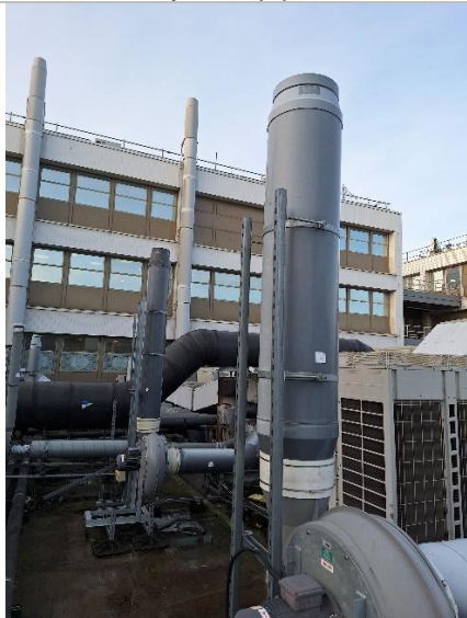
Chemistry gas flues
