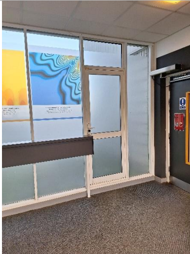
Roof access door
