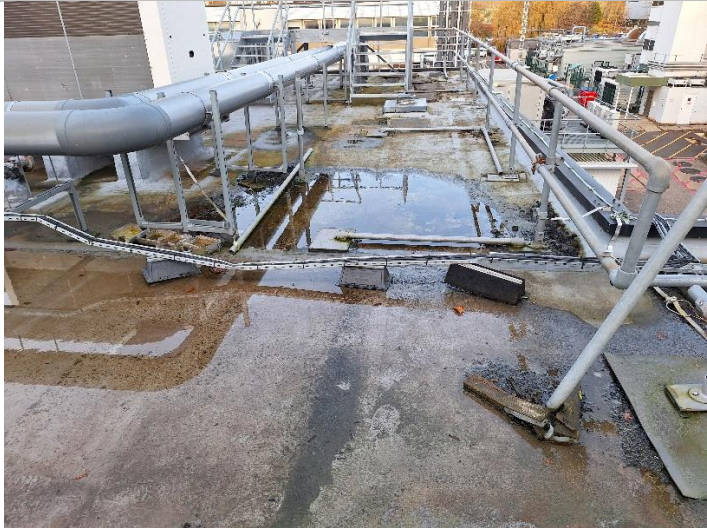
Cable tray trip hazard
