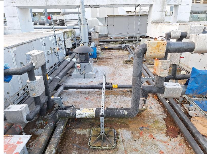
Pipework and cabling with no gantry in place.
