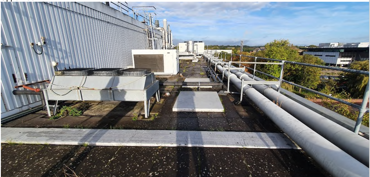
Main roof; plant and trip hazards
