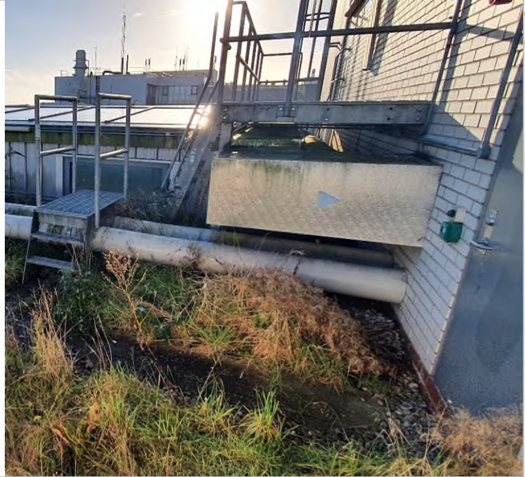
Steps onto MASB roof, ladder to upper roof and weeds on Physics roof
