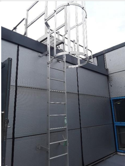
Wall Mounted steel ladder to upper-level roof
