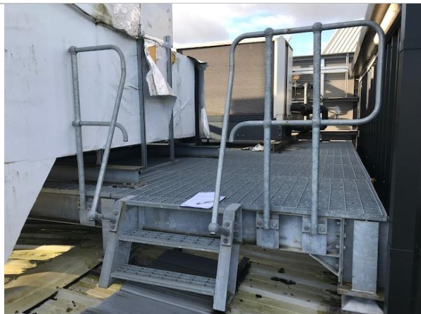
Steps on the roof housing plant and equipment
