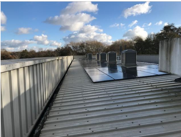
External roof with PV panels.
