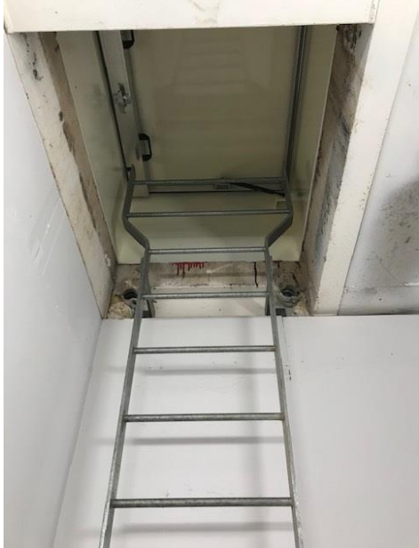
Cryfield 13 fixed galvanised ladder leading to roof hatch to access external roof.
