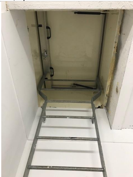
Cryfield 15 fixed galvanised ladder leading to roof hatch to access external roof.
