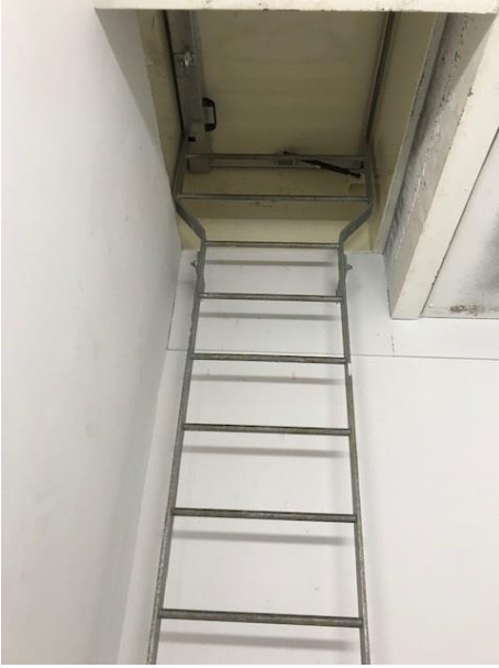
Cryfield 14 fixed galvanised ladder leading to roof hatch to access external roof.
