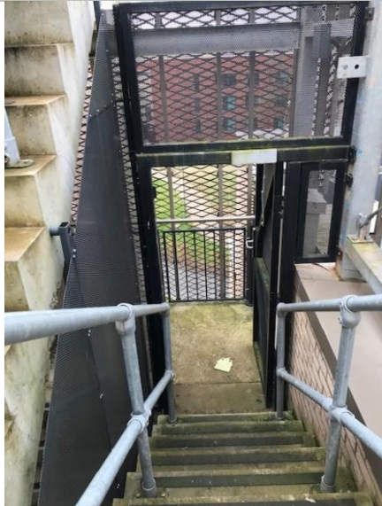
Cryfield 12 Salto access gate on the third floor.
