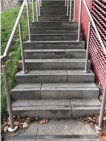
Concrete stairs leading to external access to Cryfield 10 external staircase to access roof
