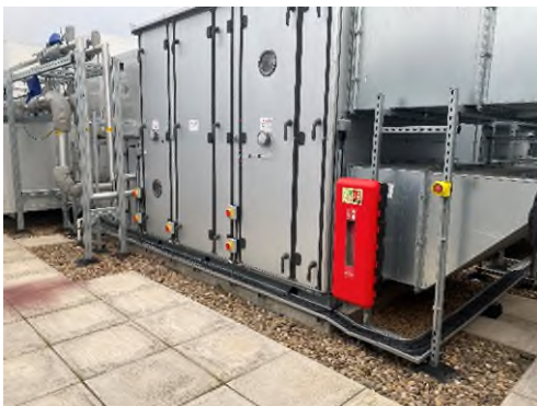
Fire detection devices and safety equipment are in place on the roof space.
