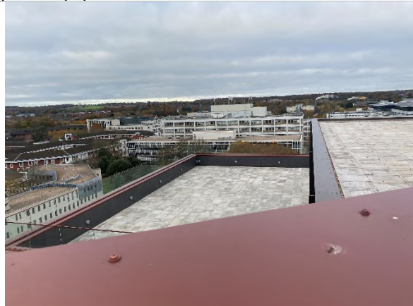
The balcony areas have edge protection/parapet walls but it is not safe to stand, kneel or lean on or use in any way as an anchor point. This should be looked at separately to any roof permit to assess any risks to working in this specific area.
