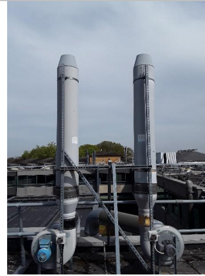
Typical Lab flues
