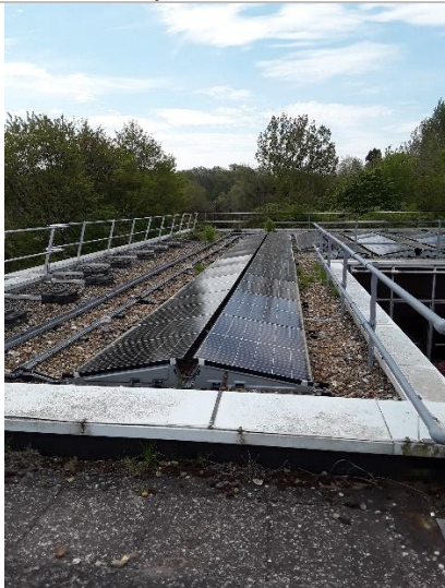
PV Panels loose ballast
