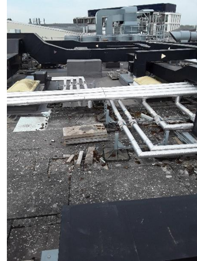
Typical pipework layout and debris
